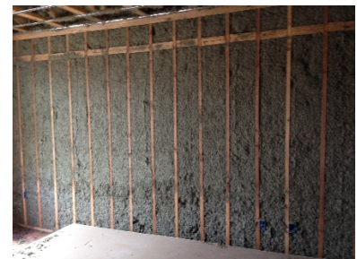
RockWool Filled Wall Cavity Fully Protecting Plumbing and Electrical
